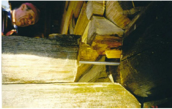
Photo 2.6: Repairing a damaged cantilever at Bakken, Bjørgum, Hylestad. The gjengestag is inserted into the beam.
