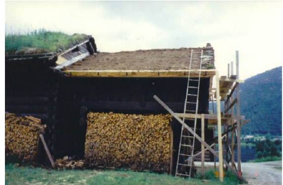
Photo 2.34: Using lead panels to protect the surface between roof/turf and timber at Bakken, Bjørgum, Hylestad.
