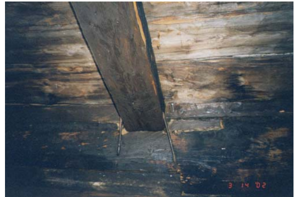
Photo 2.18: Log dogs are used to secure the rafters to the plate log (called stavlegja or raptstokken ) for stability against the wind, Tveitetunet, Valle.
