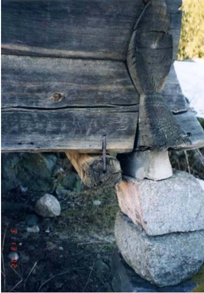
Photo 2.17: Log dogs are used to secure a sill to the beam above, loft , Tveitetunet, Valle.
