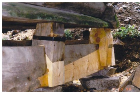
Photo 2.23: Securing a damaged leg to re-use it with the help of an iron binding on Muggslopte, at Innestog, Byklum, Bykle. See the new and replaced leg in the background.
