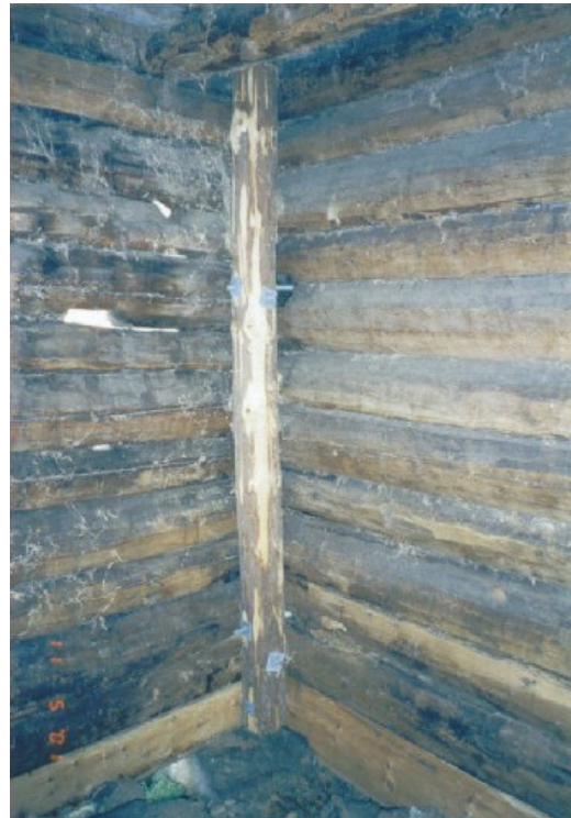
Photo 2.13: Double plank carriage seen from the inside on the barn at Bakken, Bjørgum.
