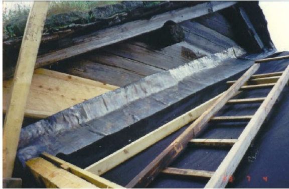
Photo 2.33: Using lead panels to protect the surface between roof/turf and timber at Bakken, Bjørgum, Hylestad.
