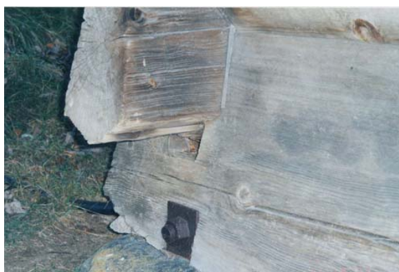
Photo 2.1: Securing a pushed out ground sill with a long gjengestag , loft , Rygnestadtunet, Valle.
