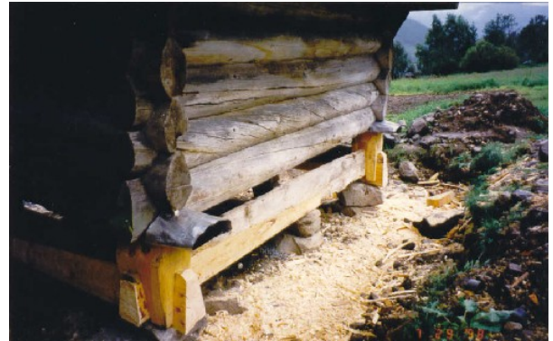
Photo 2.30: Protruding parts are covered with lead panels on Muggslopte, Innestog Byklum, Bykle.
