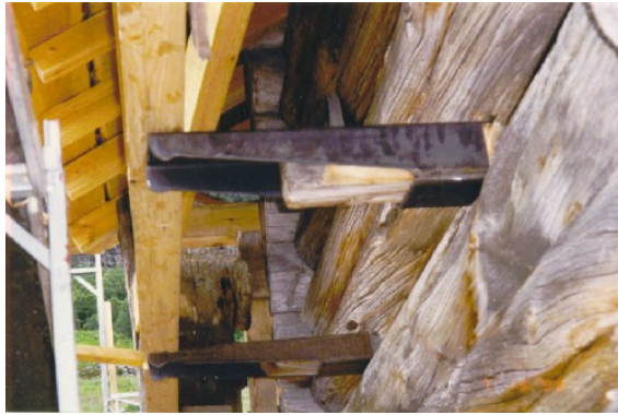
Photo 2.35: Securing the foundation in the balcony by extending the beams, Muggslopte, Innestog Byklum, Bykle.
