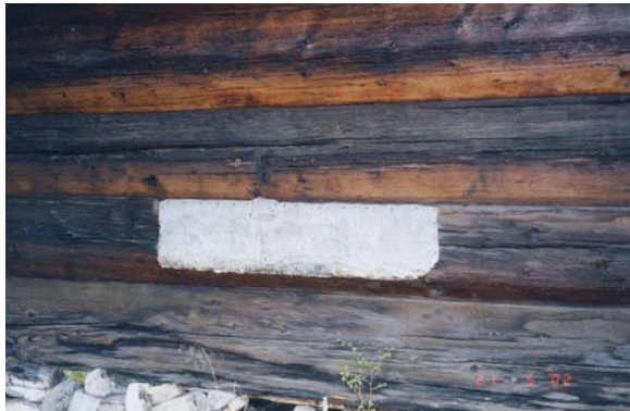
Photo 2.29: Covering up rot damage with lead panels on the hut at Henriksentunet, Bykle.
