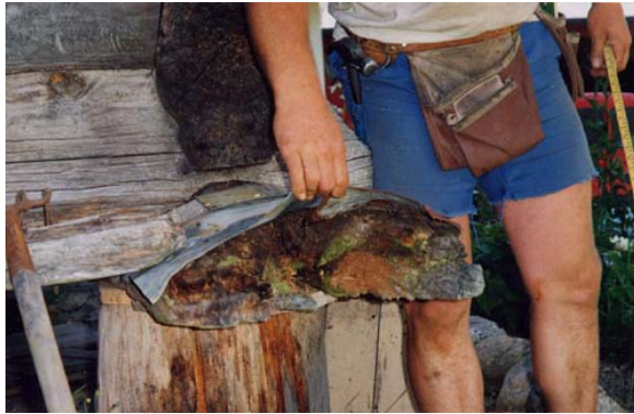
Photo 2.28: Covering up rot damage with lead panels on the house at Helle, Hylestad.
