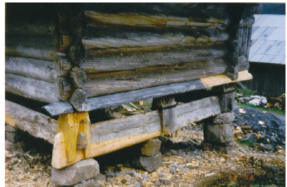
Photo 2.31: Using lead panels to secure the original sill on Muggslopte, Innestog Byklum, Bykle.
