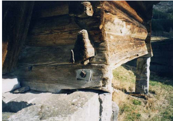
Photo 2.2: Securing a pushed out sill with a short gjengestag , Nistog Rygnestad, Valle.
