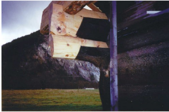
Photo 2.9: Rot-damaged cantilevers are spliced according to antiquarian methods on a loft at Dale, Valle.
