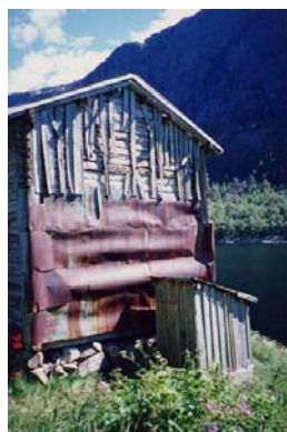
Photo 2.32: Covering rot damage with lead panels, barns at Brotteli, Bykle and Helle, Hylestad.
