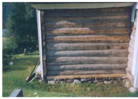
30. Chancel: Wall YC. Dismantled external panels. Bunged up rot damaged sill with new material.
