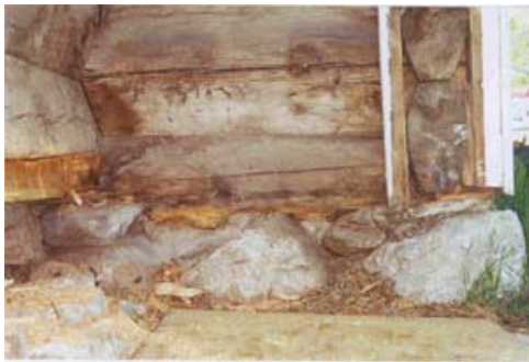
18. Nave Gable - end walls: Wall Y. Dismantled external panels. Rot damage was found on sill and corner.
