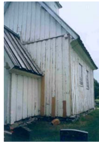
14. Nave Gable - end walls: Wall III. The photo shows the use of new wood materials - scraped and painted.
