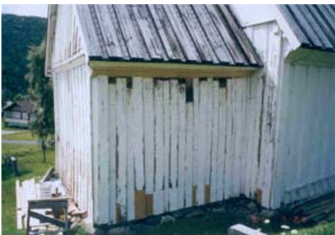
33. Chancel: Wall YC. Photo shows use of new materials. Scraped and painted.
