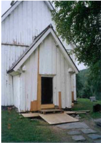
3. Entrance vestibule: Installed external panels. Photos shows that new materials were used.
