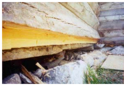
32. Chancel: Wall YC. Rot damaged sill.
