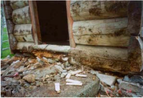
1. Entrance vestibule: The door sill had extensive rot damage.
