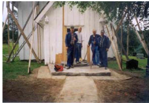
10. Stairs: The flagstone in front of the door is the original, the flagstones lie in crushed rock.
