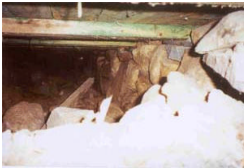
15. Nave Gable - end walls: Wall III. Joists were impregnated against parasites during the last restoration. There is no rot damage on these.
