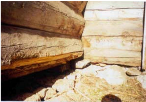
31. Chancel: Wall YC. Rot damaged sill.
