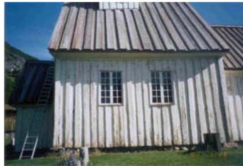
16. Nave Gable - end walls: Wall III. Attached single panels with hand-forged nails. Scraped and painted.
